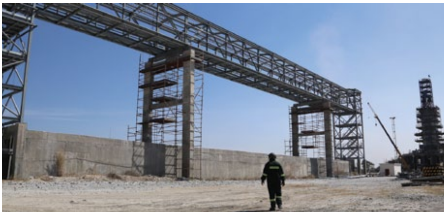
The phase 2 plant construction resulting in significant capacity increase. Photo courtesy of Ndola Lime.
