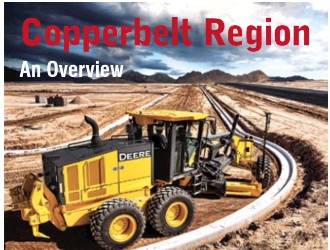
A motor grader builds infrastructure in Katanga Province, DRC. Photo courtesy of DEM Group.
